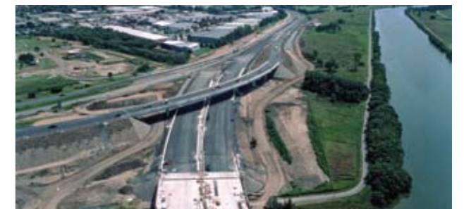
A new flyover bridge under construction at Banyo will provide access to the existing Gateway Motorway from the new Motorway.
