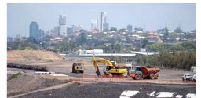
Two million cubic metres of fill and embankment materials have been transported into the site.
