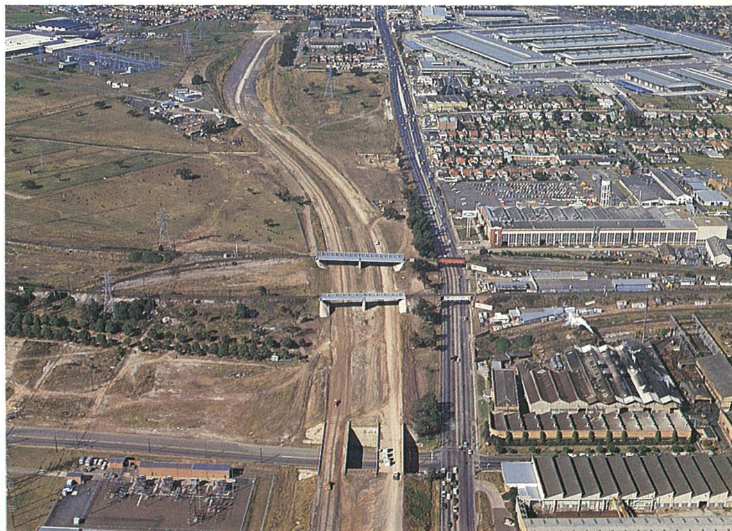
Construction of four lanes of the F4 — Western Freeway between Homebush and Clyde, adjacent to Parramatta Road.
