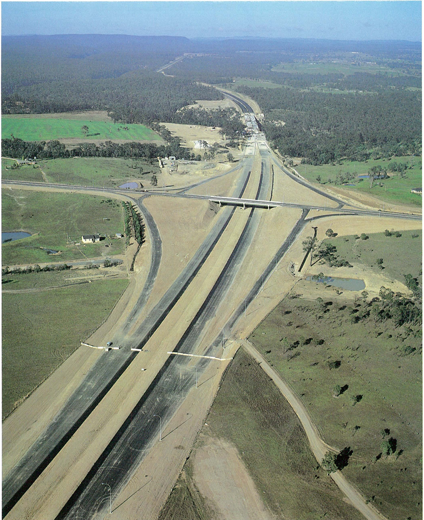
Final stages of work on the Wilton interchange which links the freeway with Maldon, Picton and the Hume Highway to the west, and with Wilton, Appin and the Princes Highway to the east — August 1980.
