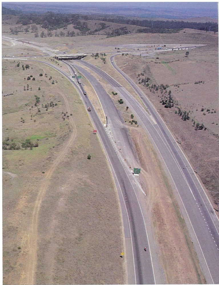
An aerial view looking south, showing construction of the Camden Road interchange.
