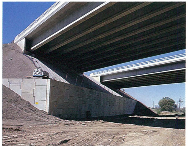
The reinforced earth retaining wall at the northern abutments of the Glenlee railway bridges.
