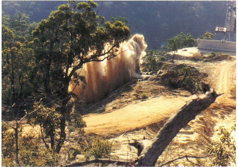
Careful blasting and earthworks operations ensured minimum effect on the natural environment.
