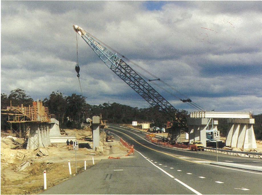
Pacific Highway access was maintained during the building of these bridges at Kariong Interchange.
