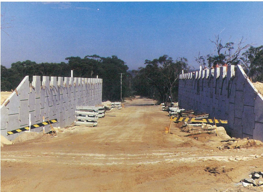
Reinforced Earth walls form the abutments of the twin freeway bridges over Gindurra Road.
