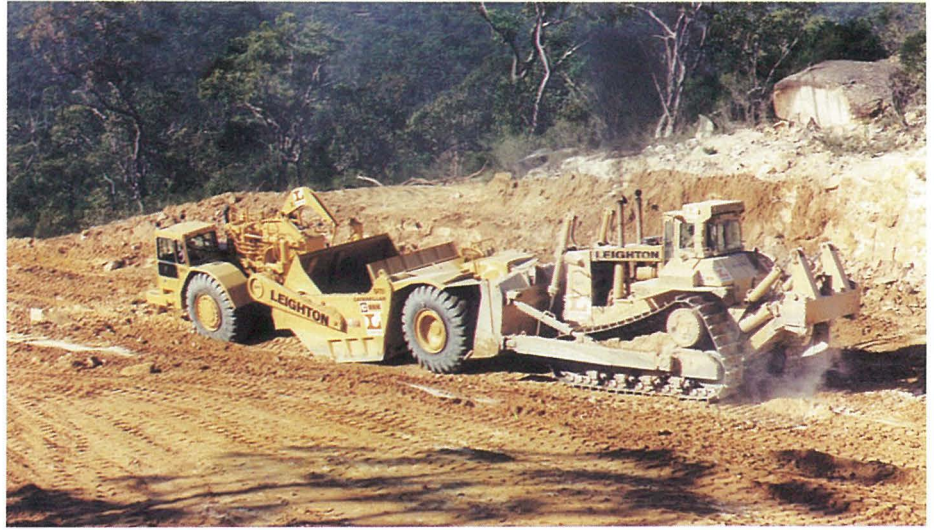
Construction contractors used some of the largest earthmoving equipment available in Australia.
