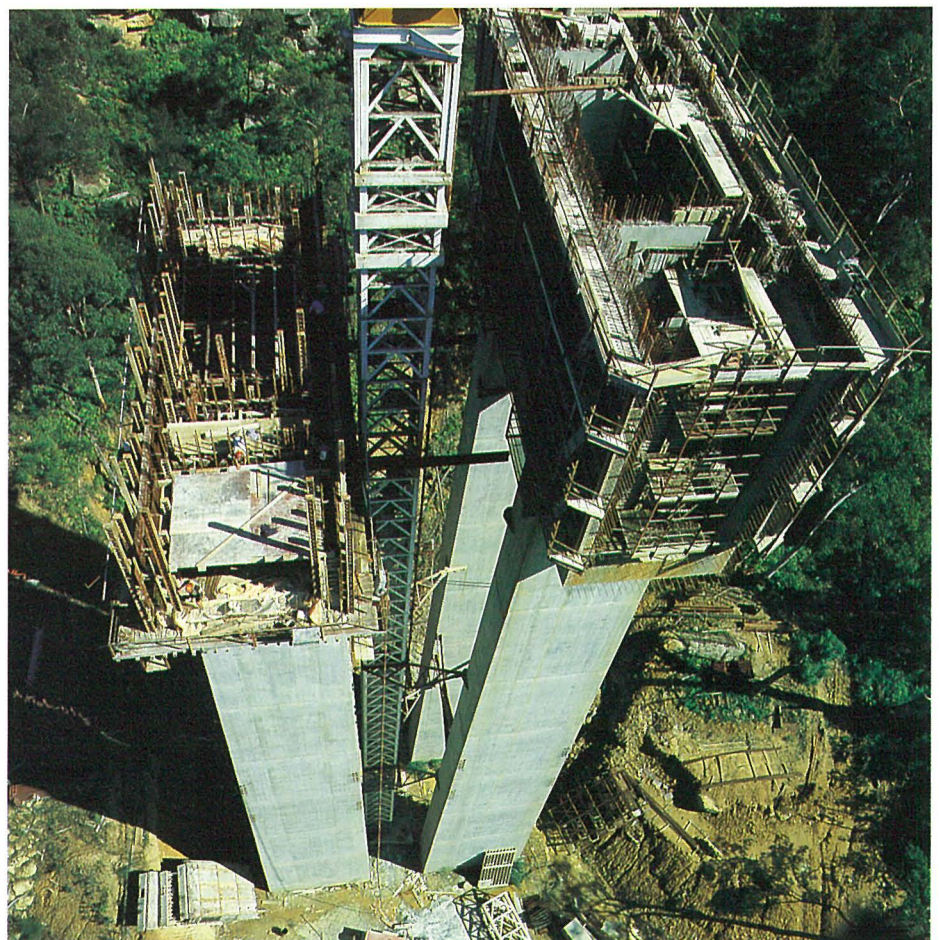
Birds-eye view of construction of piers as at March 1984, showing twin-blade design.
